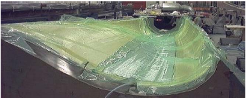
Figure 9 Set-up for resin infusion test of a root-end section of a large rotorblade at LM Glasfiber, Lunderskov, Denmark (25).
